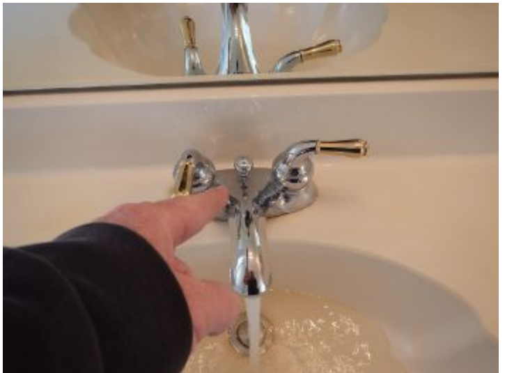
Left master vanity drain stopper needs to be adjusted
