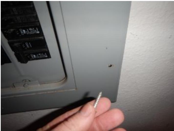
Pointed screws for service panel are not recommended
