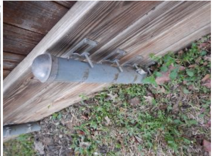
Retaining wall for fence is missing alot of hardware
