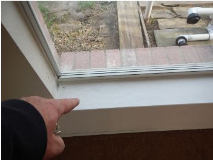
Master window is swollen and needs repair
