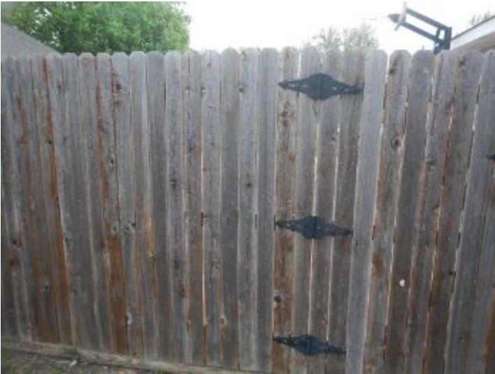
Cosmetic hail damage to fence in several areas
