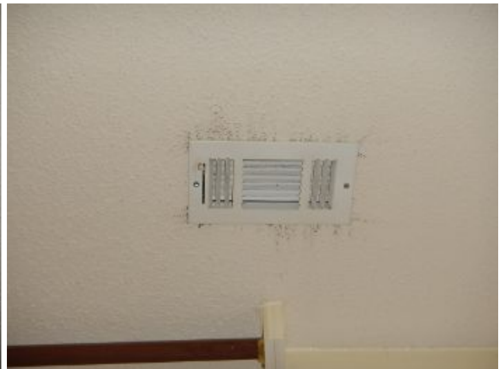
Several dirty supply vents should be evaluated
