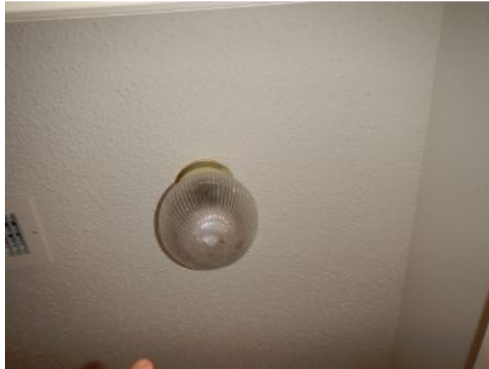
Hall bath light not working
