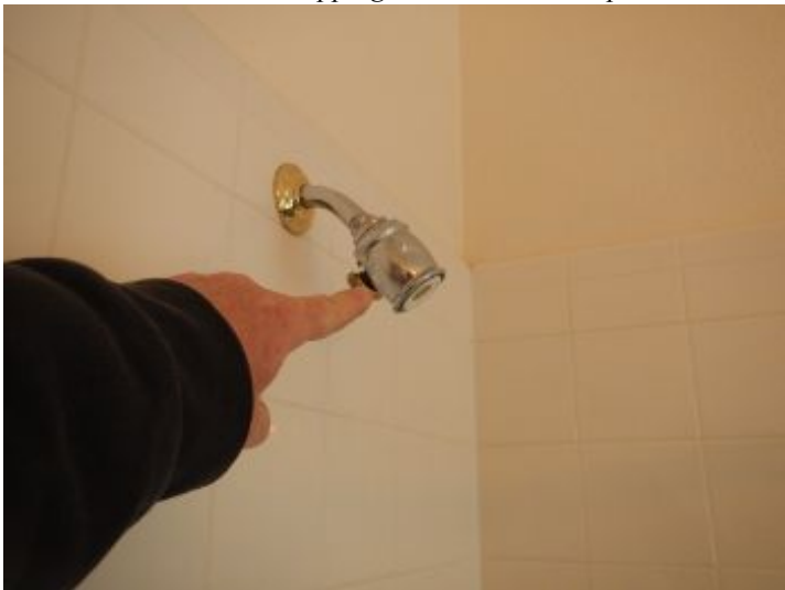
Master shower is dripping at time of inspection
