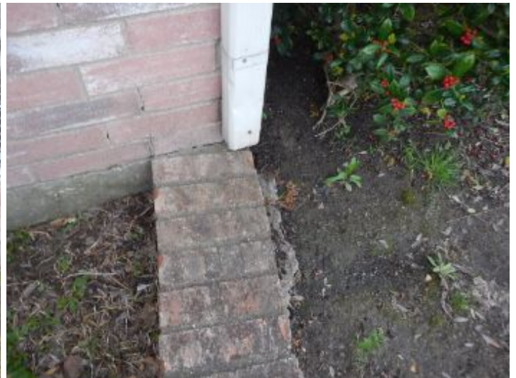
Missing gutter downspout diverter
