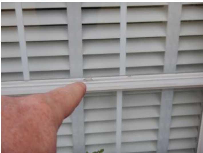
Several windows have damaged trim strips
