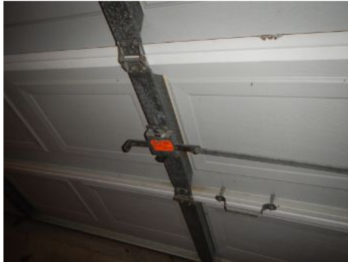
Manual locking devices should be terminated with an automatic opener
