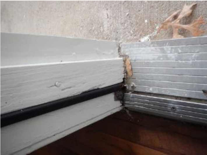
Wood rot at base of door jamb
