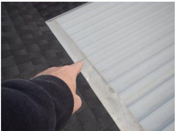
Flashing over patio cover should be sealed
