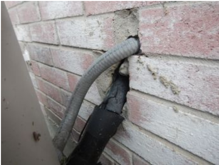
Outdoor lines need to be covered and sealed at home
