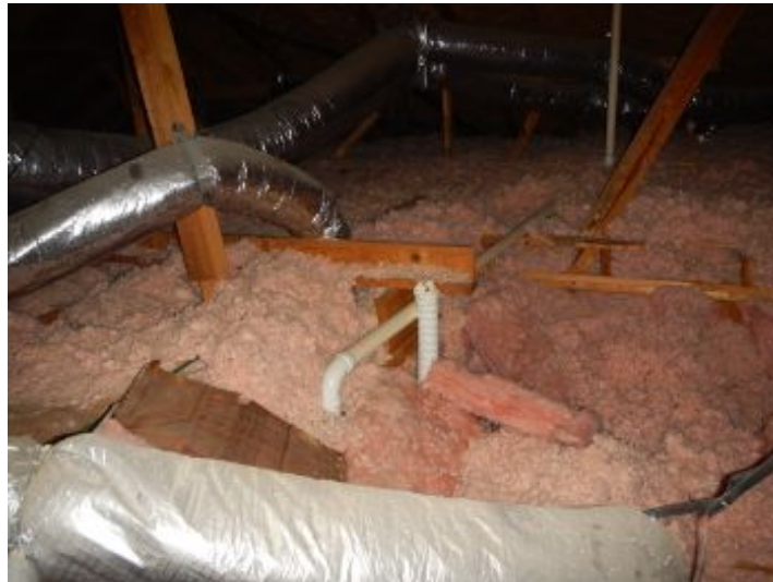
Bathroom exhaust dump into attic space
