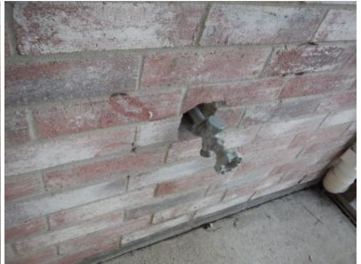
Back porch faucet needs to be properly sealed
