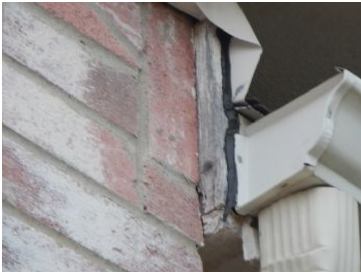
Wood rot on several fascia boards of home
