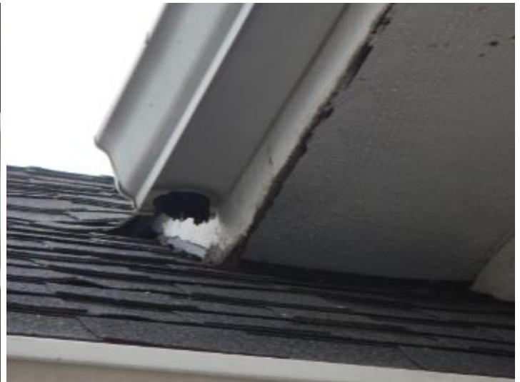
Wood rotten fascia boards needs repair
