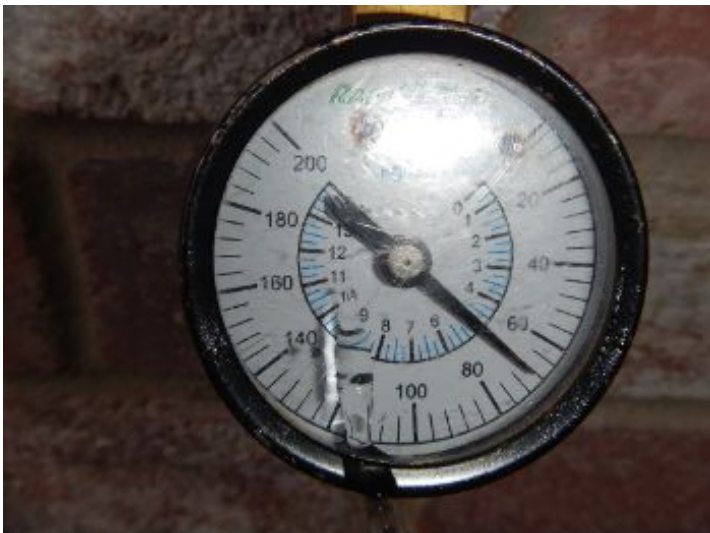
70 psi static water pressure
