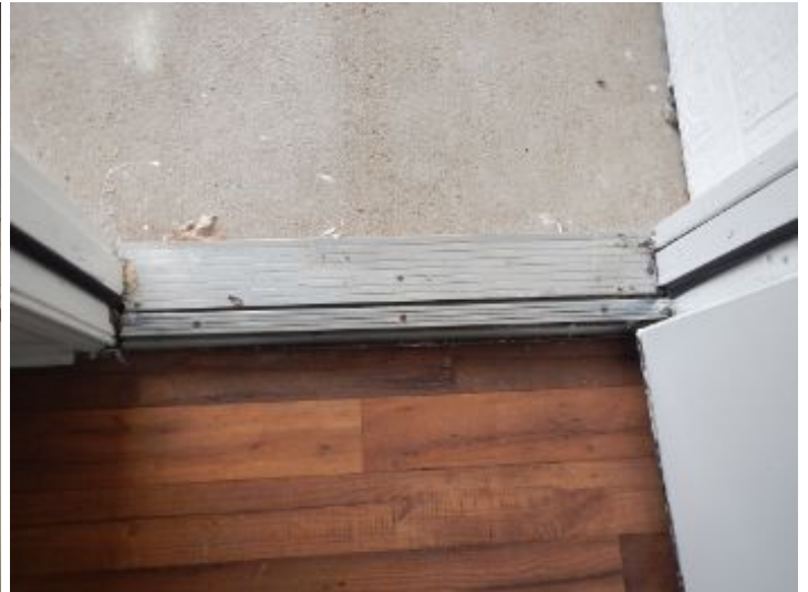
Back door to patio has a loose threshold
