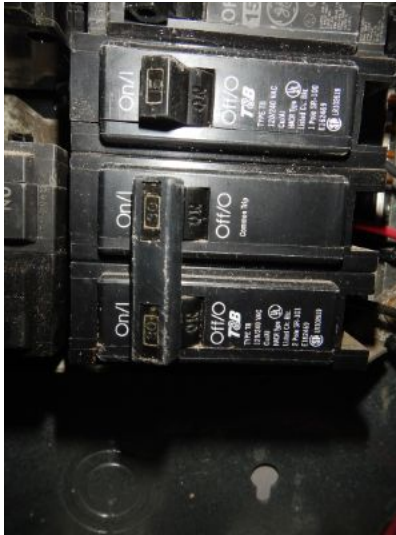
Breakers are not GE brand in panel
