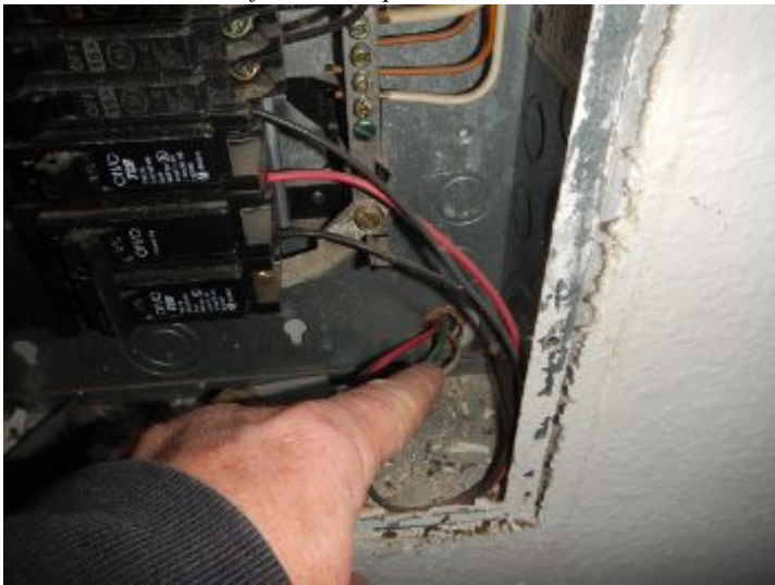
Grommet missing on service panel for exterior
