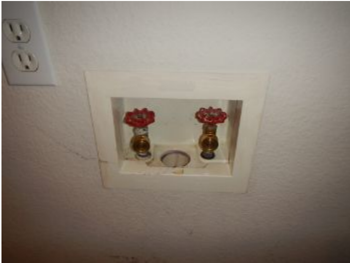
Both hot and cold faucets are leaking
