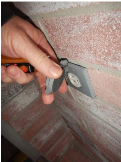
Damaged outdoor cover on front porch
