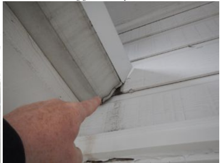
Gutter appears to be leaking above back door to home
