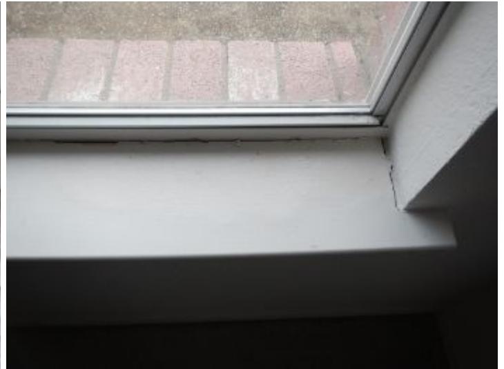
Several window sills are swollen and need repair
