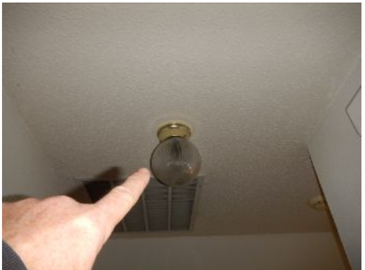
Hall light fixture was not working at time of inspection
