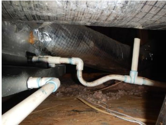
Condensation lines at unit need to be insulated
