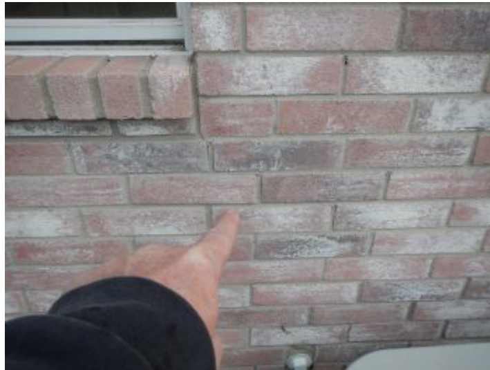
Small step cracks in brick on both sides of home
