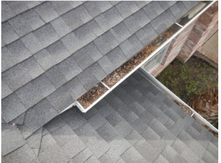
Several gutters are full of debris
