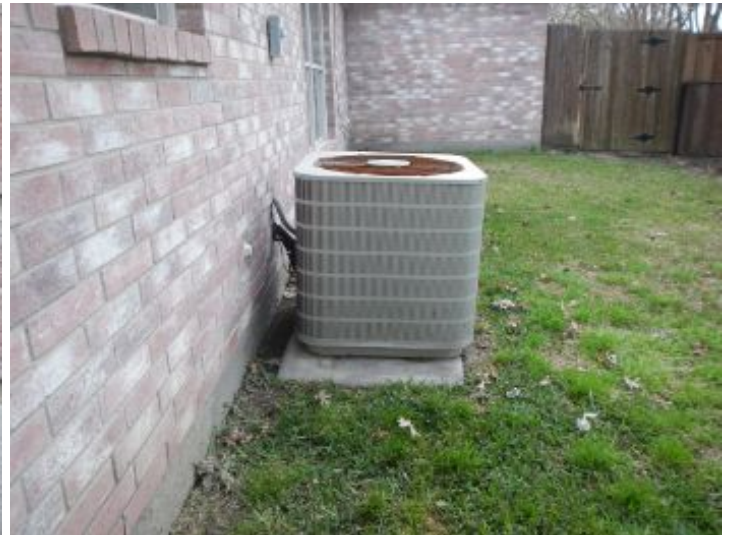
Unit is out of level at time of inspection
