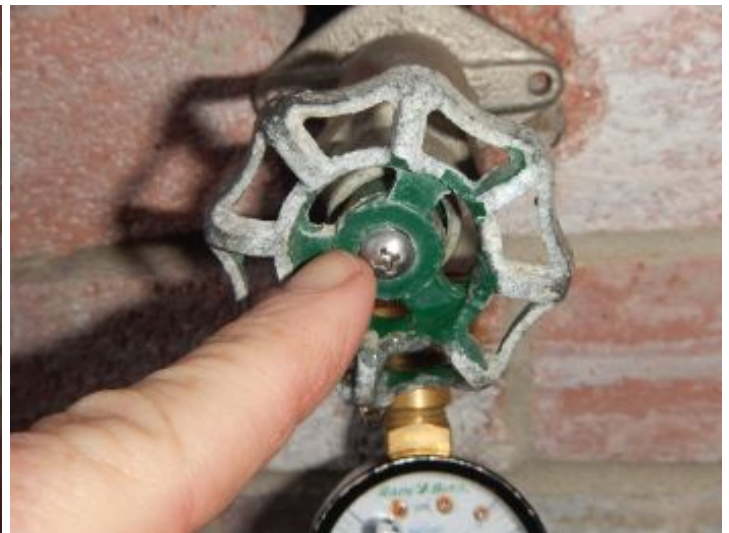
Front faucet leaks when under pressure
