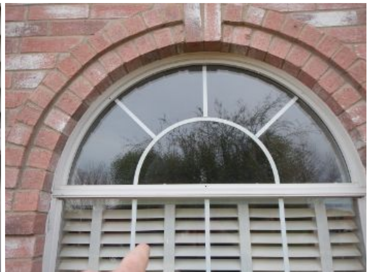
Formal room window is fogged and needs repair
