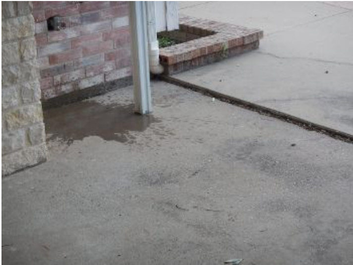
Possible drainage issue due to heaved concrete
