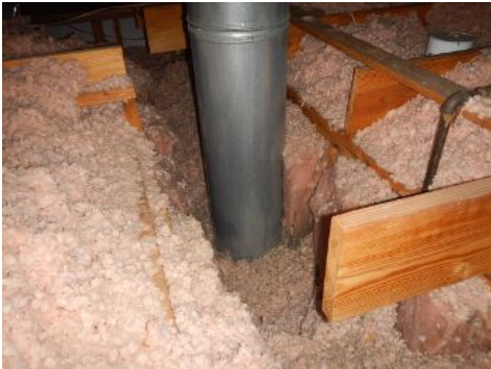
Chimney flue should be free from insulation in attic space
