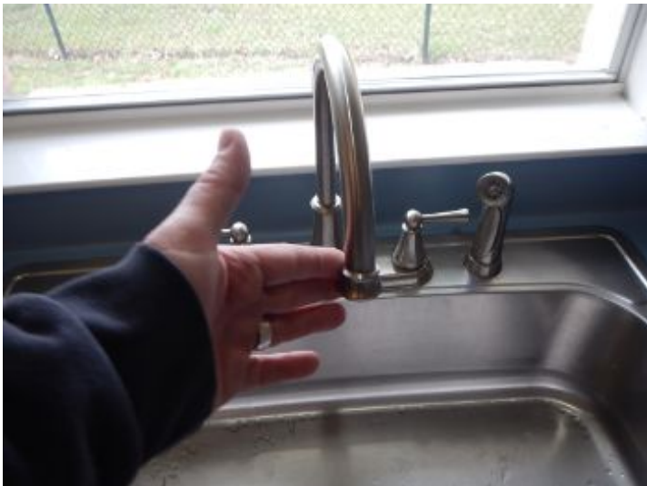
Kitchen sink is dripping and needs to be repaired
