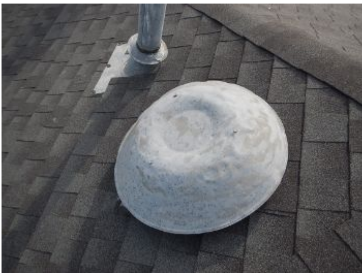
Cosmetic damage to roof vents on home
