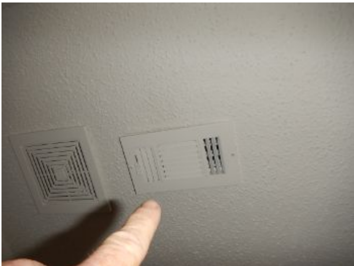
Hall bath supply register is loose at ceiling
