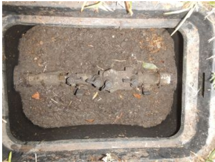
Irrigation double check was shut off at time of inspection
