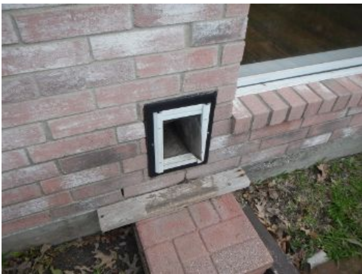
Pet door is compromised and needs repair
