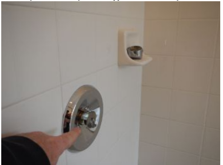
Master shower handle was removed prior to inspection. This should be repaired
