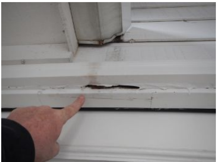
Trim around back door is rotten and needs repair
