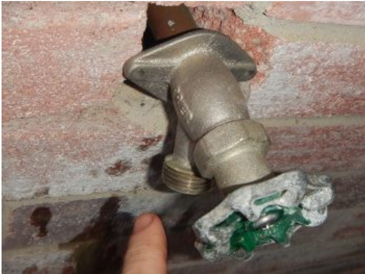
Missing frost preventer should be installed
