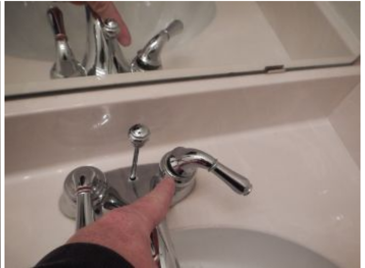
Right vanity in hall bath is loose and needs repair
