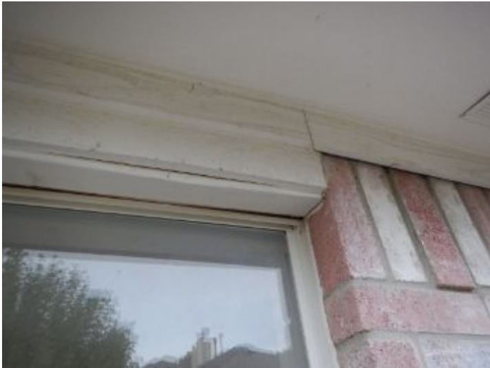
Several windows need to be sealed around
