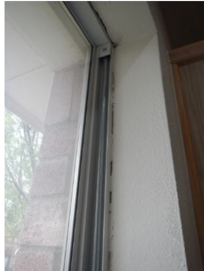
Seal around several interior windows
