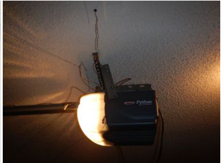
Garage door opener was not working
