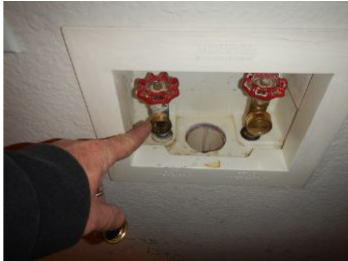
Hot and cold water valves appear to both be leaking
