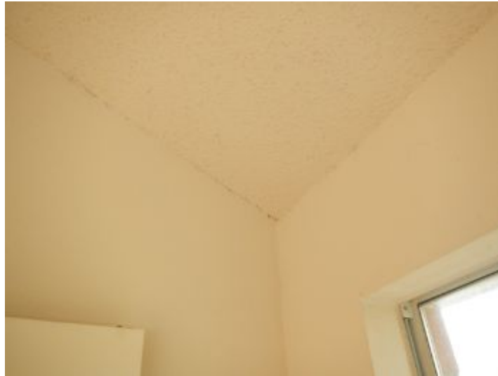
Several cracks in ceiling of home appear cosmetic at time of inspection
