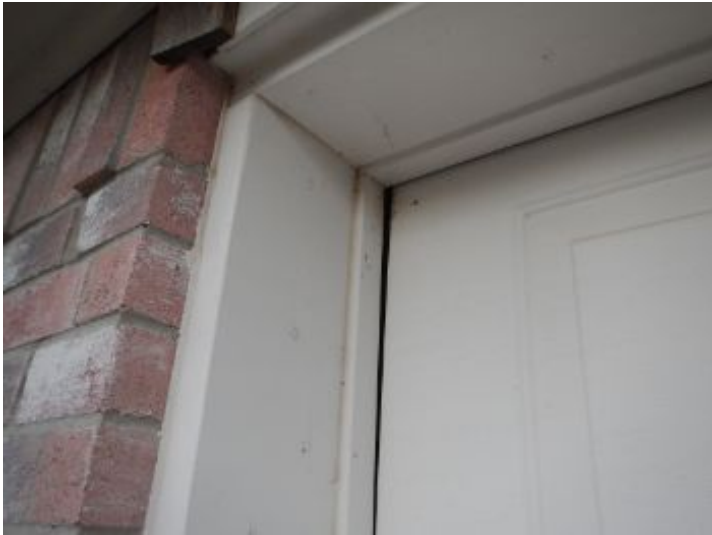
Garage door appears out of align at time of inspection
